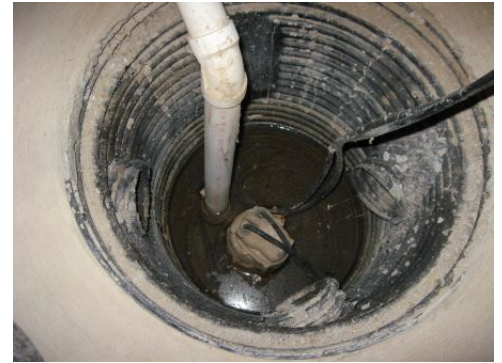
Figure 6.30: A sump crock.
